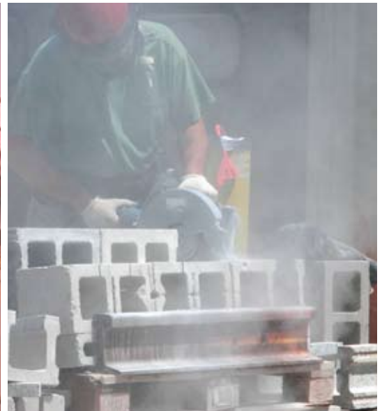
Incorrect way to cut masonry.
